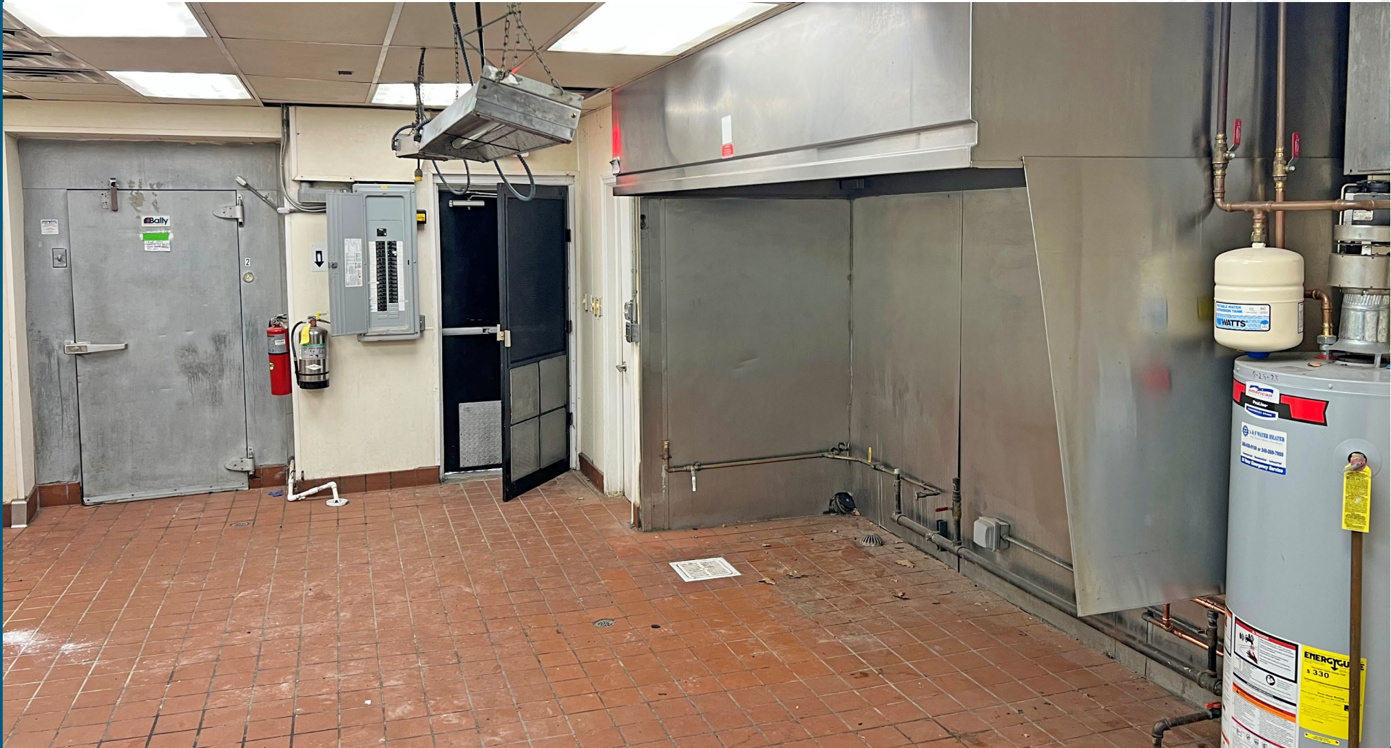
EXISTING RESTAURANT LAYOUT AND INFRASTRUCTURE IN PLACE
